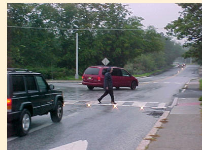
Crosswalk with in-pavement flashing warning lights installed and operating at the time of the third evaluation
