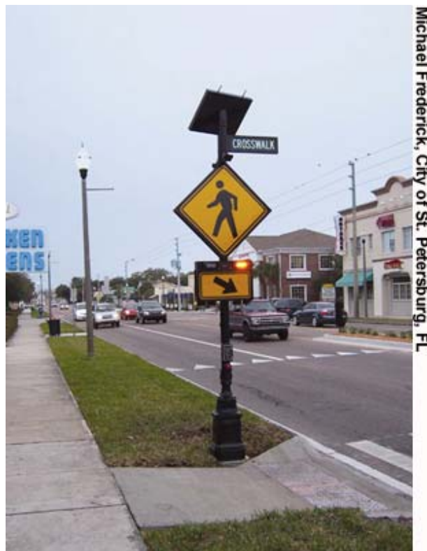
This photo shows a closeup shot of the RRFB installation on U.S. 92 in St. Petersburg, FL.
